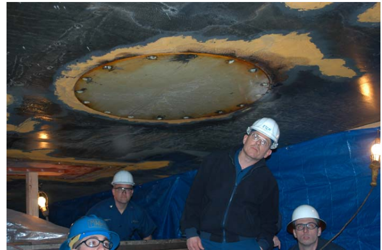
2. Well of the 75-kHz phased array ADCP
